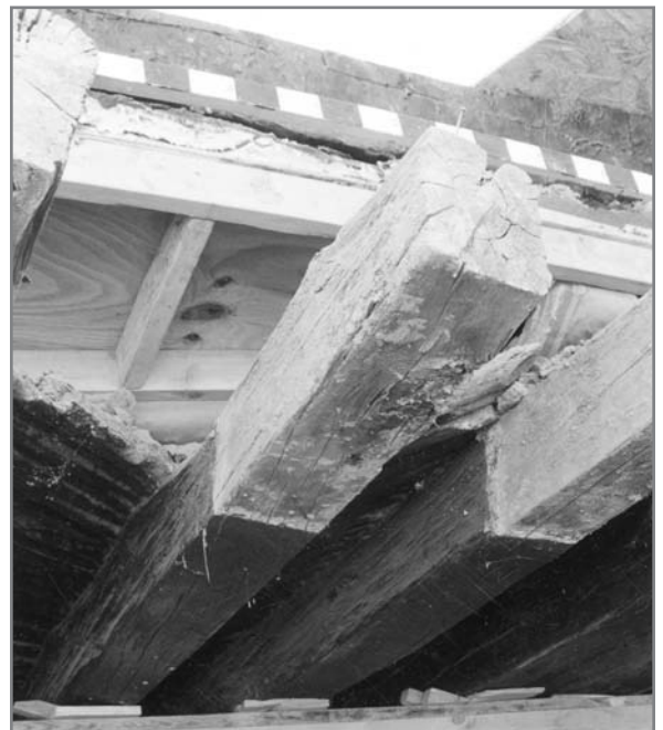
Before and after photos of deteriorated vigas repaired using the viga splicing method (Method D).
